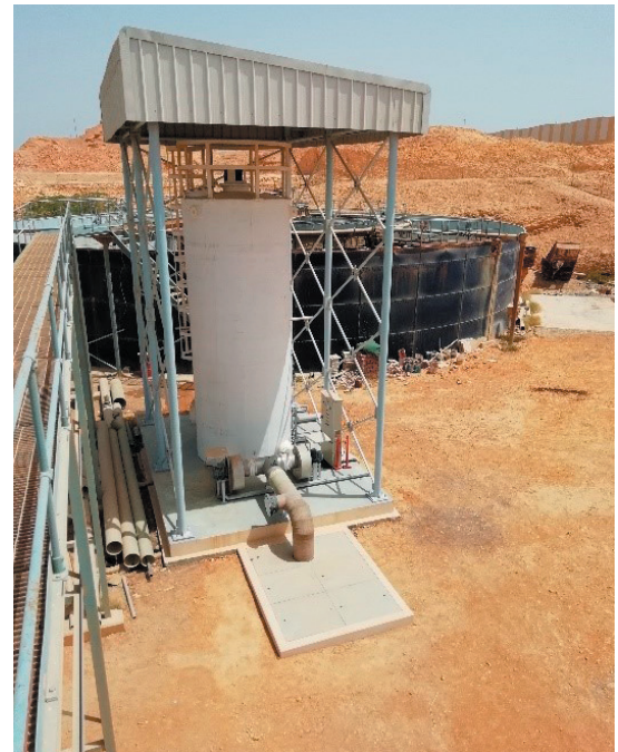
Biotrickling system at Rusayl Industrial Estate (Oman)
