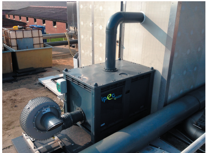
Corrosion Control for H_2S & NH_3 Removal (Manure Treatment – Belgium)
