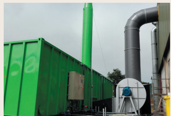
Odour Control on municipal waste sorting plant (Ireland)
